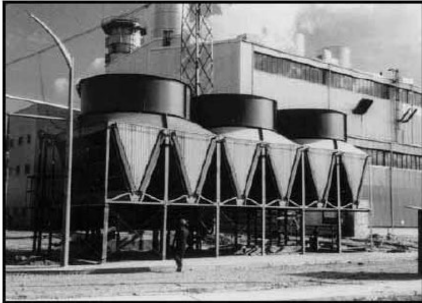
Figure 1.3.3 is a picture of auxiliary dry/wet cooling cells. Id.
