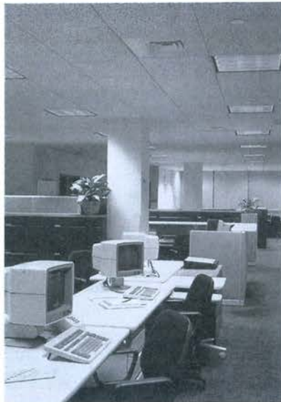
Figure 26-5. An ambient lighting system that also provides wall and task lighting.
