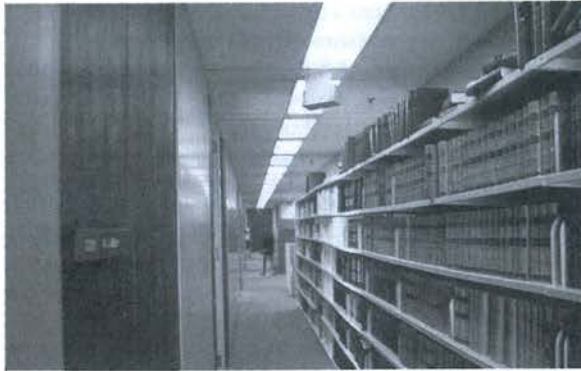
Figure 29-5. Overhead troffers, some of which are supplied with emergency power, are aligned with the path of egress to more conspicuously delineate the path.
