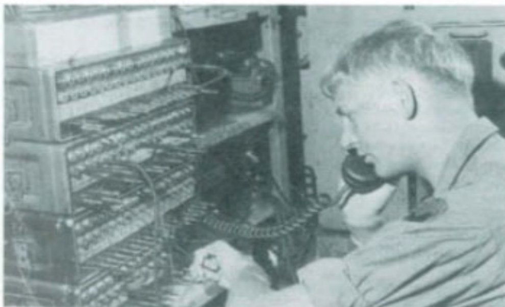
SB-22 SWITCHBOARD aboard the Benewah.
