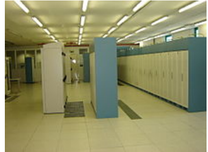
Lucent 5ESS GSM Mobile Switching Centre deployed at Western Wireless International in Ljubljana, Slovenia from 2001 to 2006.
