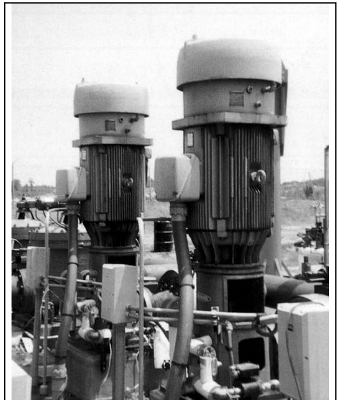
Fig. 2 Process Pump Drive Motor in a Petro-Chemical Plant
