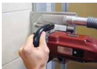
Cut into the tiled wall
