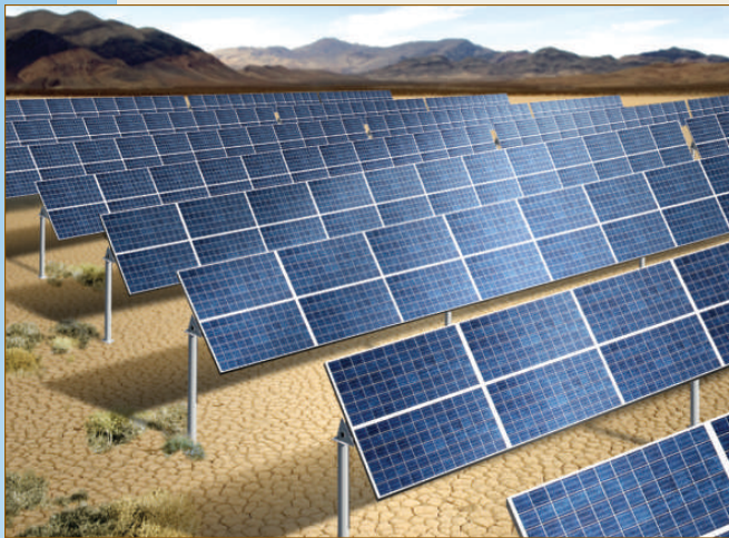
Ground-mounted RayTracker GC
