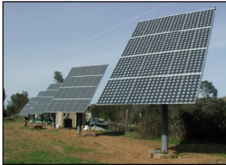
Six Wattsun AZ300 Trackers: 24 Siemens SP75 Modules per tracker. Installation by Electron Connection
