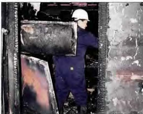
An investigator searches for clues inside the gutted living room of this single-family home, which was damaged when food left cooking unattended on an electric stove ignited.
