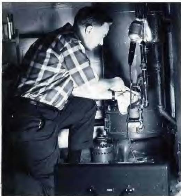
To reduce the risk of CO poisoning, homeowners should have their heating systems inspected and cleaned every year.
