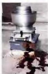
Rooftop grease creates uncontrollable fire hazards
