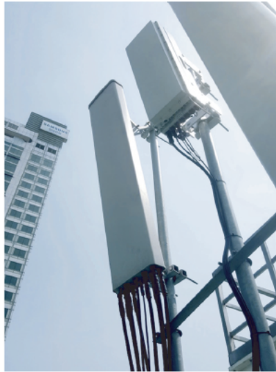
Figure 4: Co-located 32T32R and 8T8R MIMO antennas
