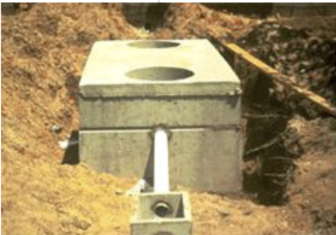
Septic tank and distribution box
