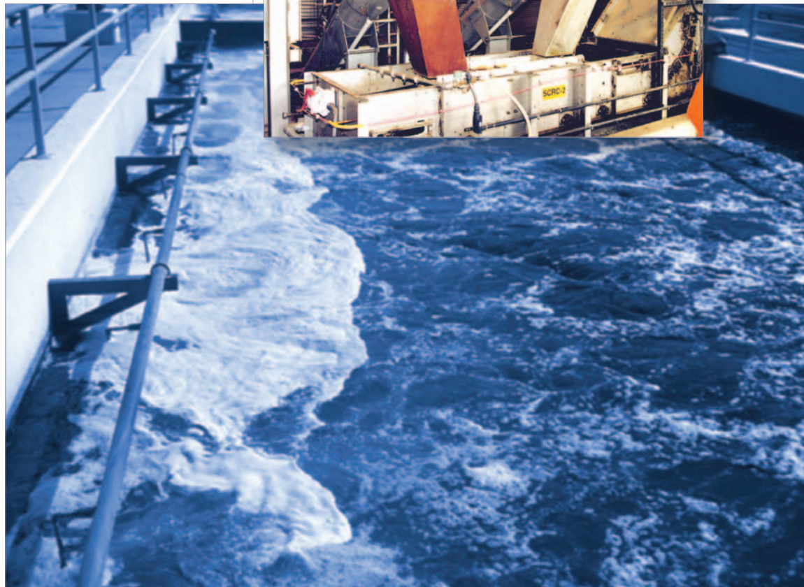
Aerated Grit Chamber
