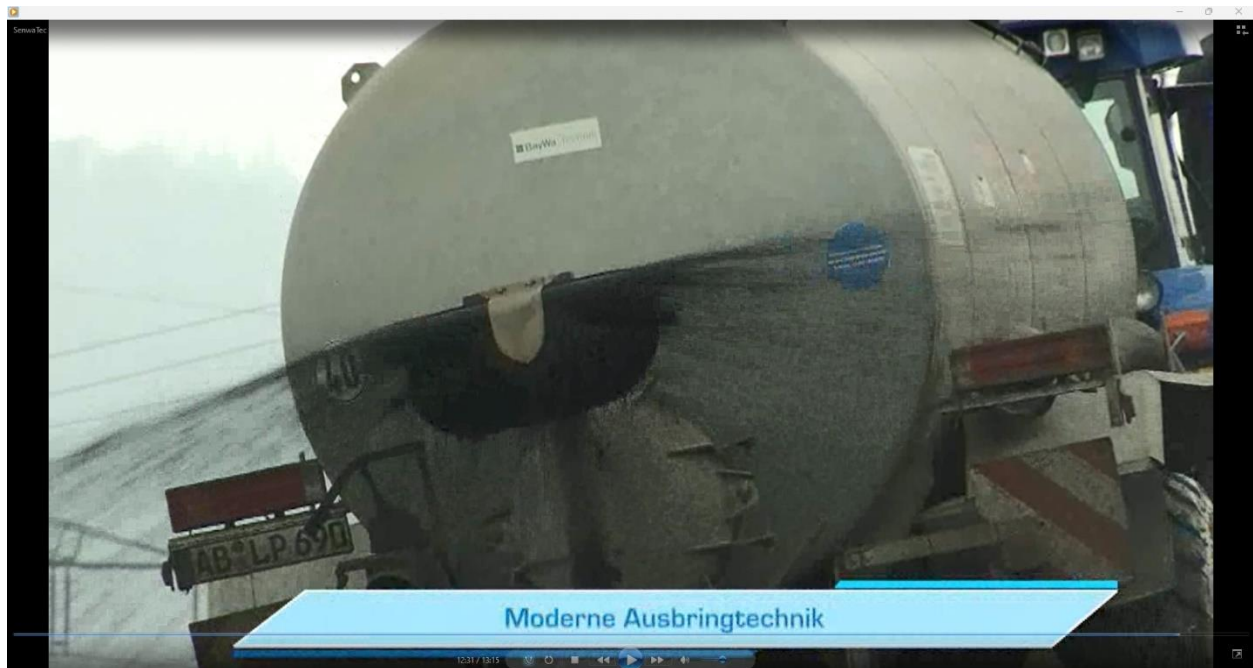
Modern delivery technology
