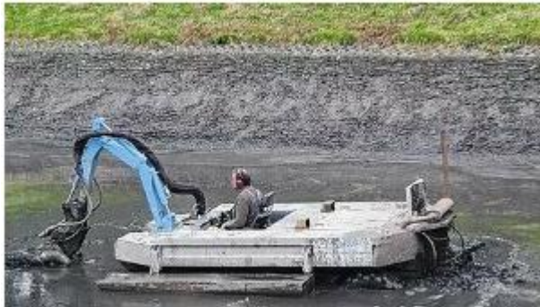
Photo: Andrea Kemmer | A stirring job: Eckhard Funk agitates the sewage slurry in the basin of the Neubrunn sewage treatment plant with his amphibious vehicle and then sucks it out.
