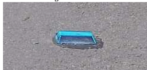
The blue reflector should be in good condition
