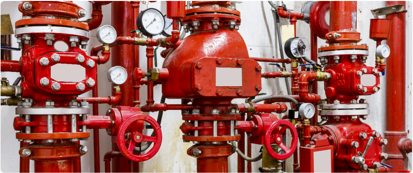
Fire sprinklers are the most effective suppression system.
