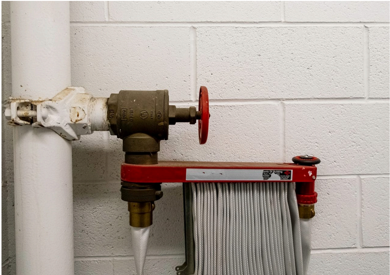
Fire House, Warehouse complex, Active fire protection (AFP) standpipes
