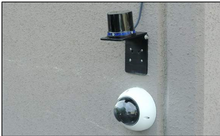
Figure 12. Wall-Mounted for Security
