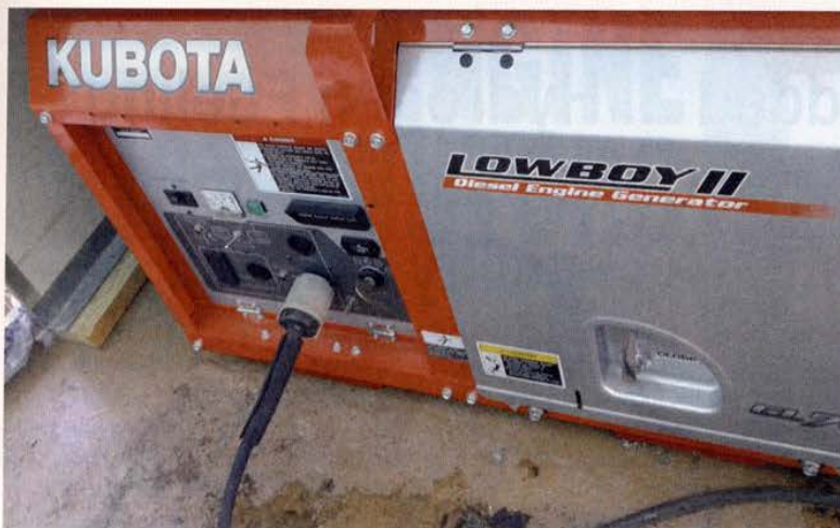
Kubota Engine America (KEA) donated a GL7000-USA Lowboy generator set to the Science Barge to allow its hydroponics and pumping systems to operate when the sun and wind don't cooperate. The gen-set, rated 7.0 kW standby, operates on B20 biodiesel.
