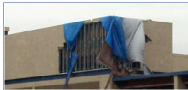
This roof tarp should have been secured by wrapping the edges around pressure-treated wood and nailing the wood to the roof.
