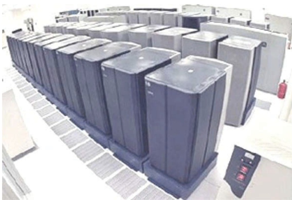
Fig. 1. Physical organization of a data center.
