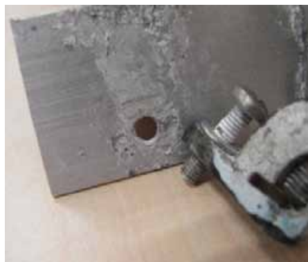
Figure 10 Build-up of white oxidations on the aluminum frame (lug sample)
