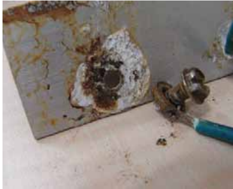
Figure 9 Build-up of white oxidations on the aluminum frame (screw sample)
