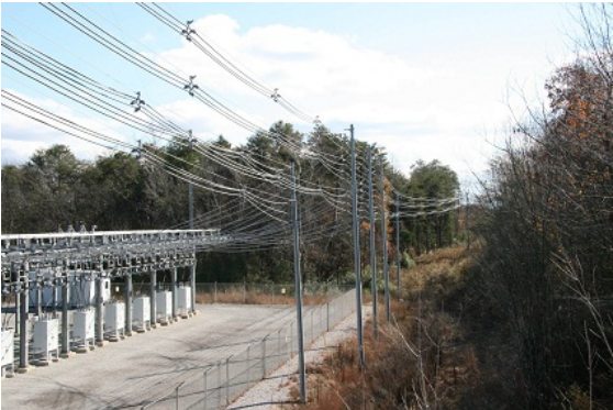
The power lines exit a substation serving a mountainous Tennessee community. Limited right of way is a big challenge when putting up new power lines because there is no way to obtain additional land for more open wire circuits.
