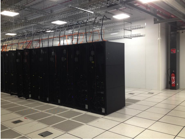
Fig. 1. Data center in Nokia, Lannion.
