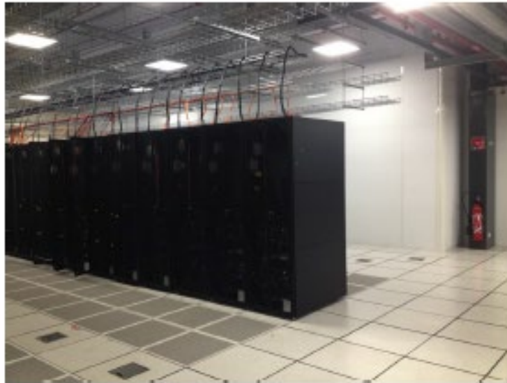
Fig. 1. Data center in Nokia, Lannion.
