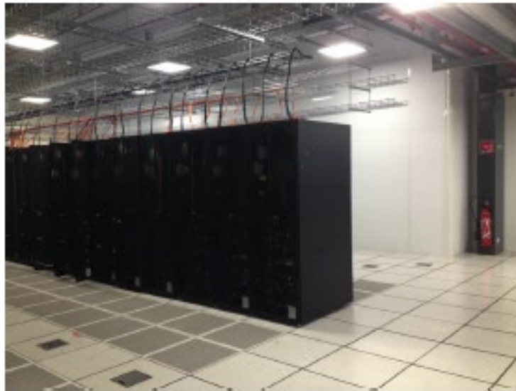
Fig. 1. Data center in Nokia, Lannion.
