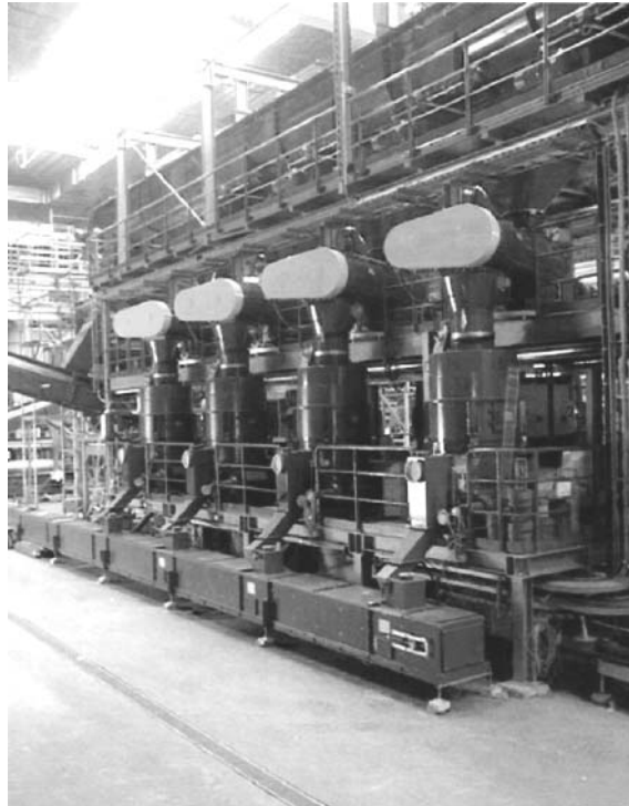
Fig. 8.36 Four flat die pellet presses of the secondary solid fuel manufacturing plant at Schwarze Pumpe, Germany (courtesy Amandus Kahl, Reinbek, Germany)
