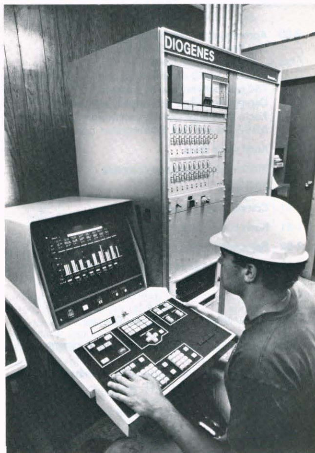
FIG. 11. Pilot plant digital controllers.
