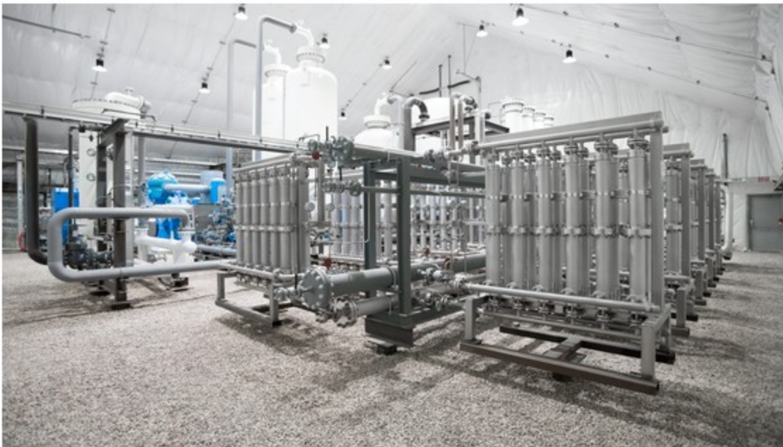
Helium membrane plant at Mankota, Canada
