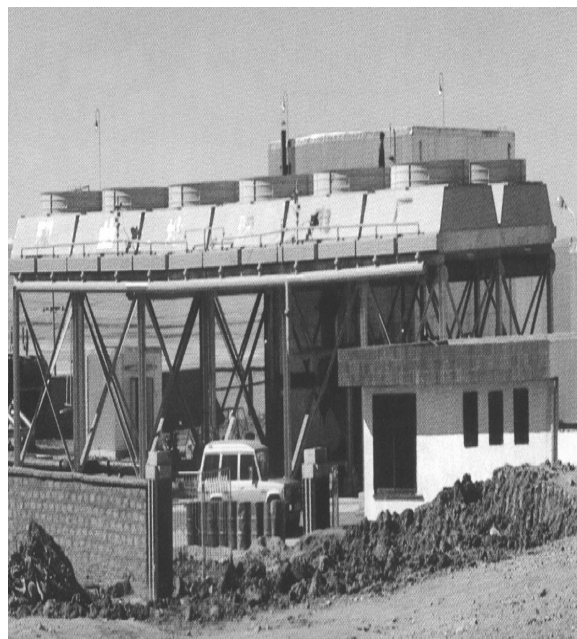
Figure 4. Nagqu 1.3 MW Air Cooled Binary Geothermal Plant
