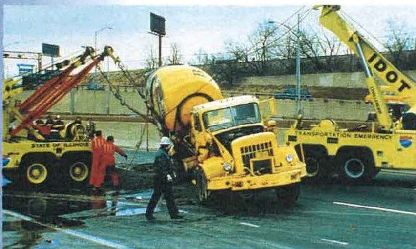
Incident management and emergency management systems often work with freeway management systems to help transportation and law enforcement officials locate, respond to, manage, and clear highway incidents promptly, thereby decreasing congestion and preventing secondary accidents.
