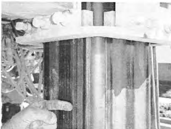
Damage caused by binding
