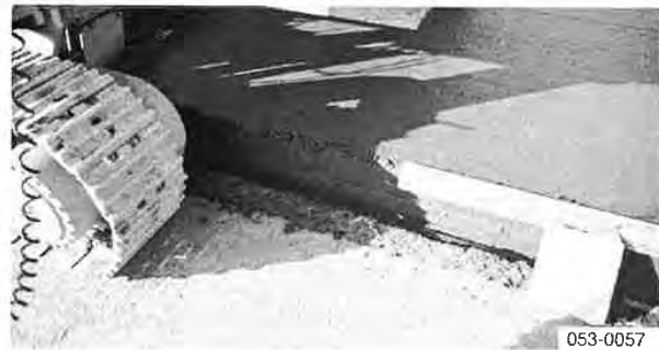
Bad edge caused by low concrete level
