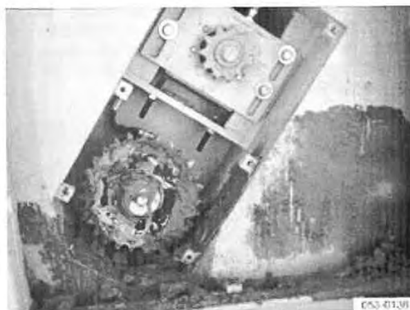
Broken drive chain
