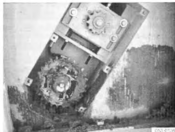
Broken drive chain
