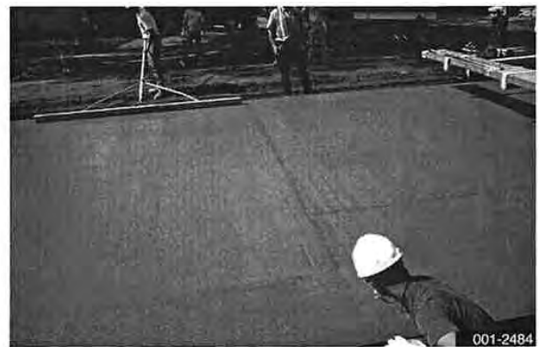
Hump caused by running vibrators
