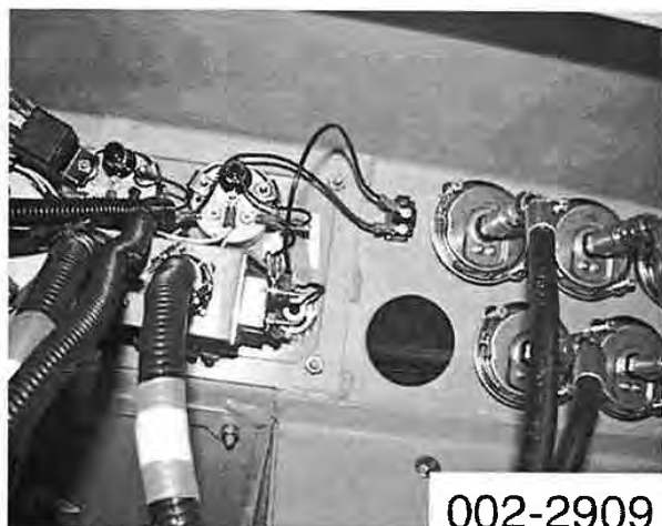
Flood light switch
