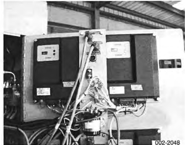
S2X controllers mounted to access door
