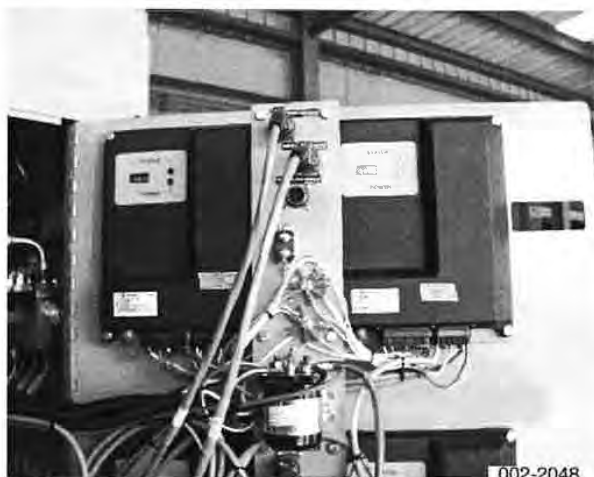
S2X controllers mounted to access door
