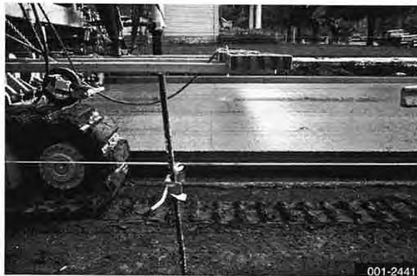
Bump caused by bumping line or sensitivity too high
