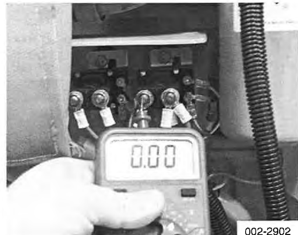
Defective starter relay
