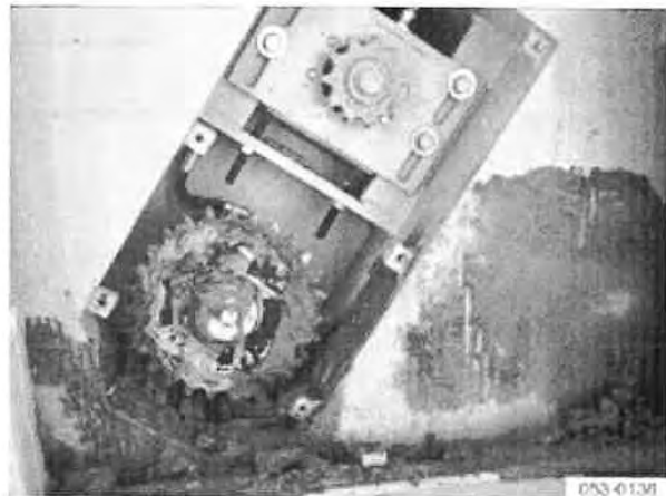
Broken drive chain
