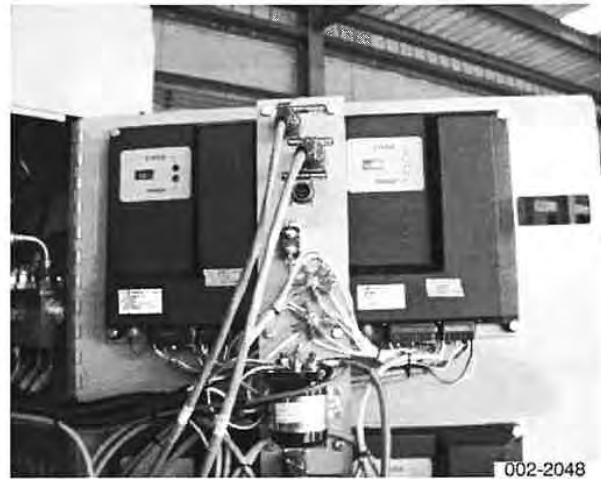
S2X controllers mounted to access door
