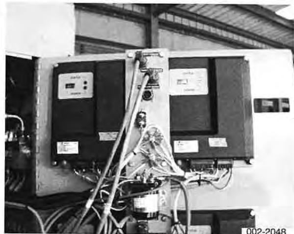
S2X controllers mounted to access door
