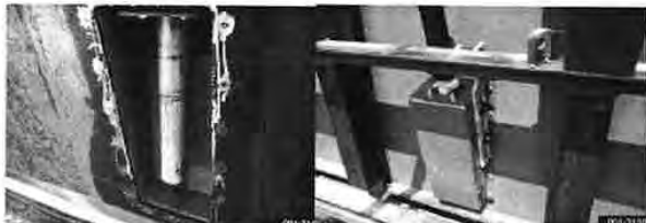
Vibrator installed in barrier wall sideplate
