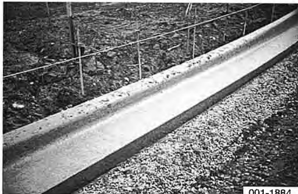
Voids in concrete surface
