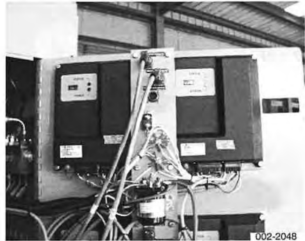
S2X controllers mounted to access door
