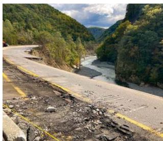
Hurricane-Damaged I-40 Through N.C.'s Mountains to Be Reopened to Traffic March 1
