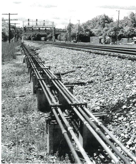
FIGURE 5.6. Mechanical interlocking pipes at Hancock Tower (Hancock, West Virginia) used to operate remote switches. Photo Credit: Michael Brotzman.
