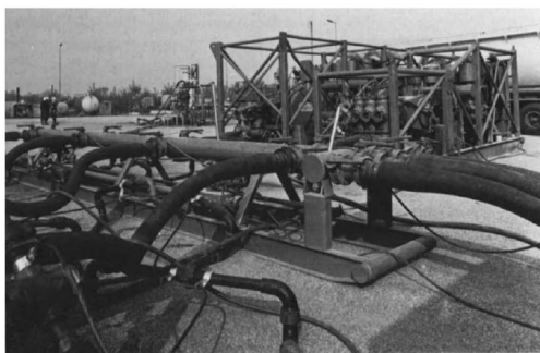
Figure 3.61 Close-up view of some of the large amount of equipment required at the well-site for an hydraulic fracturing job. (Photo: NAM)
