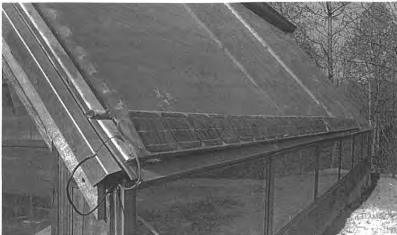
Figure A.6. Skyheat workshop-fabricated hybrid solar cell array installed on a greenhouse. (David Ross Stevens photo)
