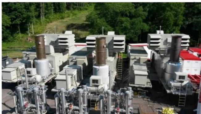
Figure 3—Three mobile turbine generators with natural gas filtration units
