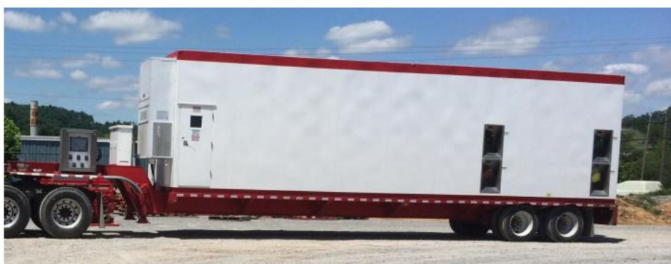
Figure 5—Switchgear for the electric powered hydraulic fracturing fleet
