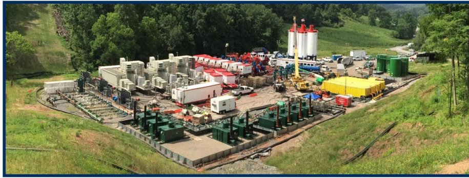
Figure 1—Electric powered hydraulic fracturing fleet in West Virginia
