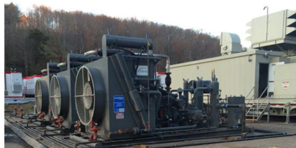
Figure 2—Gas compressors for the turbines
