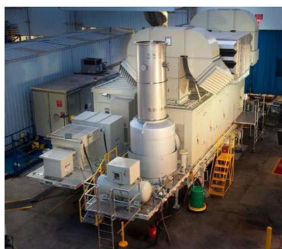
Figure 4—Turbine Engine and Generator Trailer and Electronic Equipment Room Trailer
