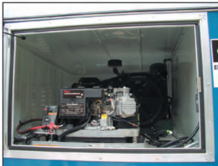
Gas Powered Generator
