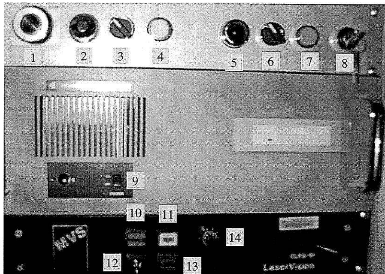
Figure 6-3. Front panel of controller cabinet, 1: emergency shutoff switch, 2: motor controller power indicator light, 3: motor controller off/enable switch, 4: motor controller on indicator light/push button, 5: linear slide power indicator light, 6: linear slide off/enable switch, 7: linear slide on indicator light/push button, 8: master power switch, 9: computer power switch, 10: laser controller power push button, 11: laser controller test push button, 12: laser controller master switch, 13: laser indicator light, 14: laser current control knob
