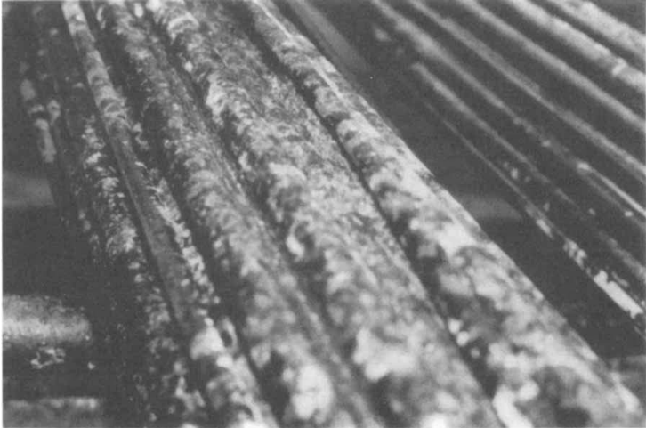
FIG. 1. Fouling on the shell side of an ammonia reactor effluent cooler operated with treated cooling water.
