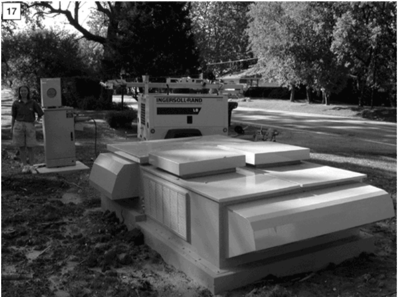
Above ground portion of a buried controlled environment vault (CEV). A portable generator is attached to a power box in the background
