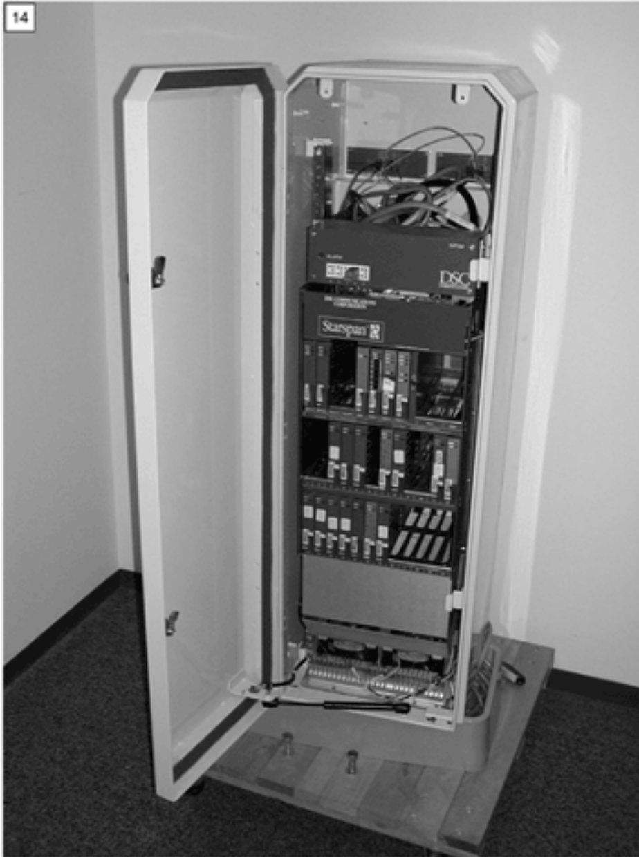
An opened optical network unit (ONU) able to serve 96 lines (laboratory model), about 1 meter tall.
