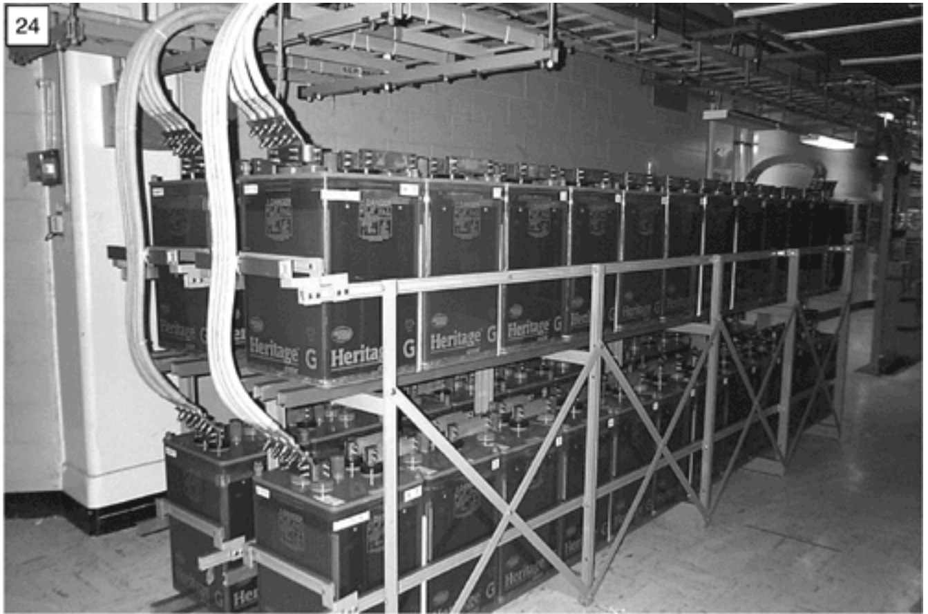
A portion of the 8 hour reserve battery
