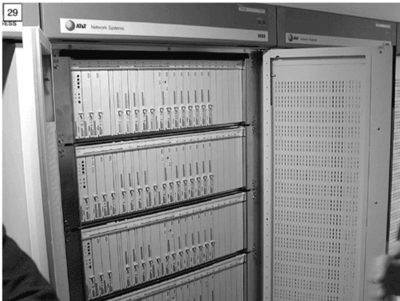
5ESS™ switch voice line unit
