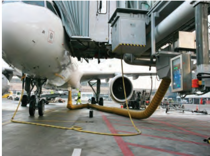
Figure 39. Aircraft connected to PCA hose and ground power cable at gate (Source: Zurich International Airport).
