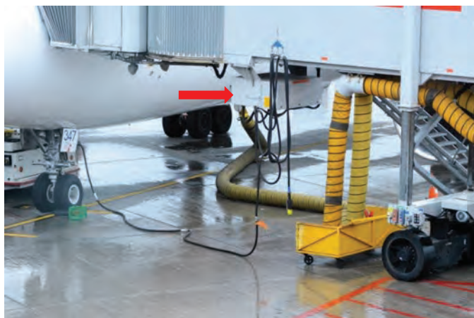
Figure 4. Aircraft connection to ground power (black cable) with frequency converter (red arrow), and PCA hose (yellow ribbed hose).
