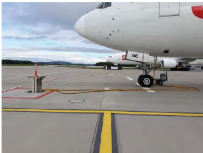
Figure 16. 400 Hz ground power underground pit system (Source: Fleuti and Ruf 2018).
