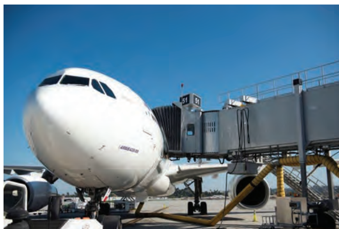
Figure 33. PCA and GPU connection at SAN jet bridge (Source: San Diego International Airport).
