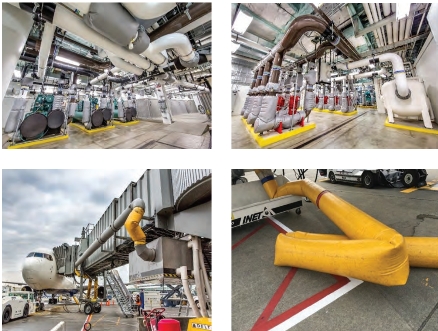
Figure 35. Clockwise from top left: Ice storage in central plant, central plant pumps, kinked PCA hose, and aircraft connected to PCA and ground power (Source: Port of Seattle).
