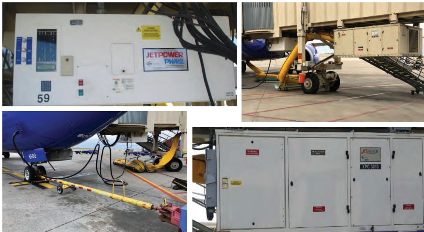
Figure 26. Clockwise from top left: 400 Hz ground power unit, aircraft connected to the PCA unit, 30-ton PCA unit, and aircraft connected to the 400 Hz ground power unit (Source: Jerome Cowart, ABM).
