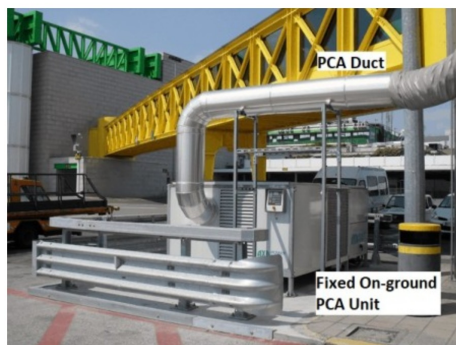
Fixed on-ground PCA units can have their duct elevated and run under jet bridge tunnels exiting just near the aircraft (Image Source: ITW GSE)
