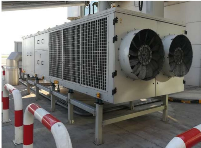
An electric PCA unit runs on utility power supply received from airport building
