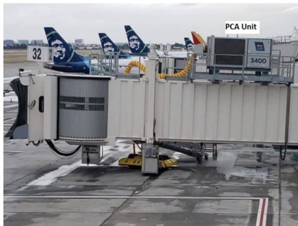
Sometimes, PCA units can also be mounted over the jet bridge instead of hanging under it (Image Source: ITW GSE )
