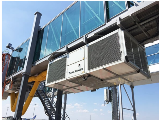
Bridge mounted PCA units cannot be easily serviced or maintained because of difficulty in their accessibility without a ladder or aerial platform (Image Source: ITW GSE)
