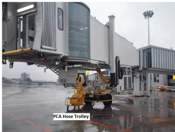
Bridge mounted PCA units have a trolley in front of jet bridge bogie to carry the PCA hose (Image Source: ITW GSE )
