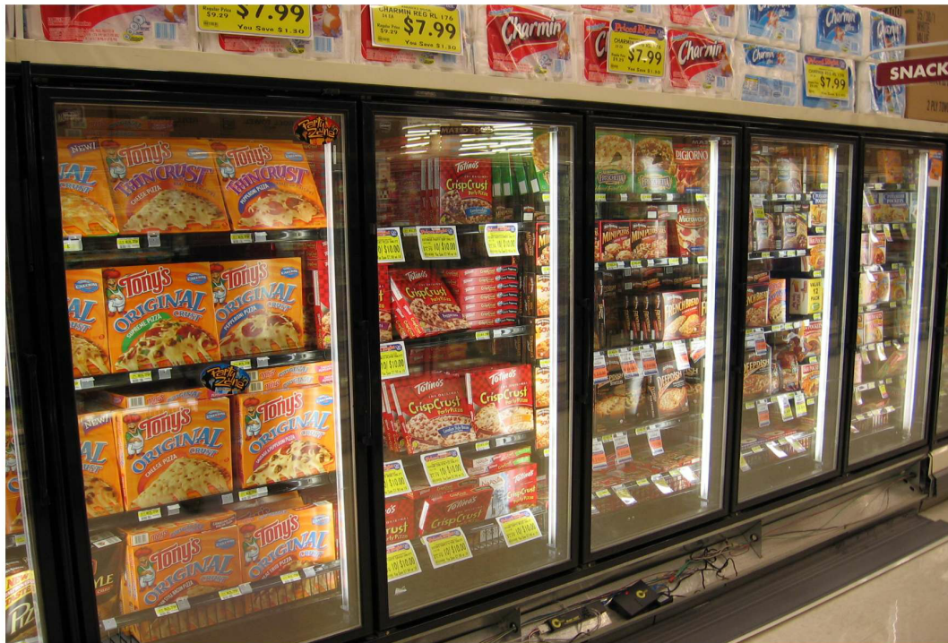
Figure 1 Refrigerated case used to evaluate ControlTec's AS-20 anti-sweat heater controls
