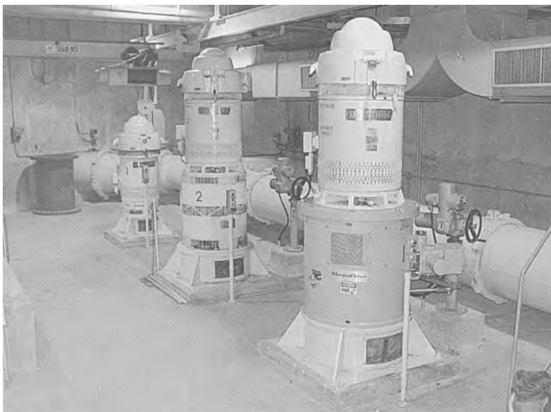
FIGURE 5 Vertical centrifugal pumps driven by a permanent magnet ASD (front), an eddy-current coupling (center), and a direct coupled motor (back) (MagnaDrive Corp.)
