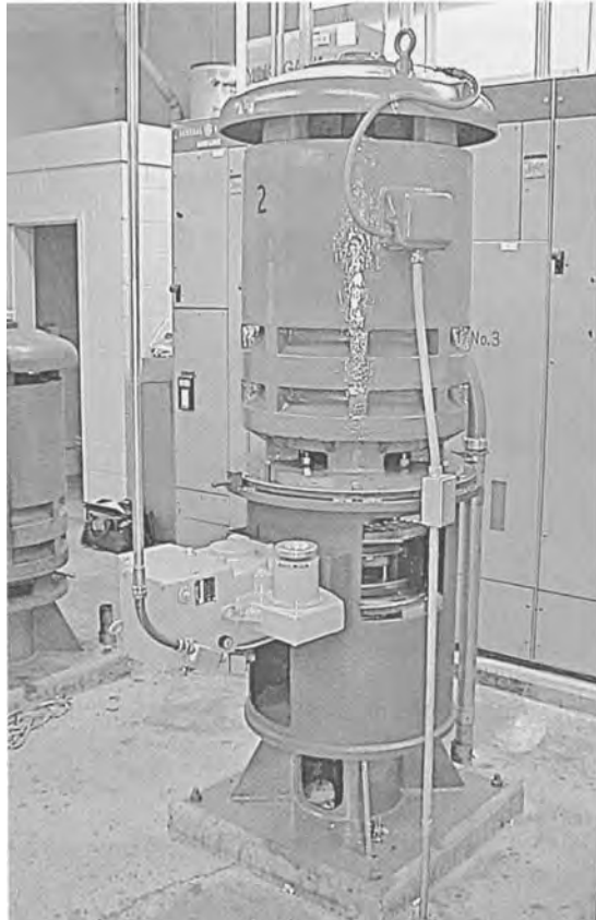
FIGURE 4 Vertical centrifugal pump driven by 350-hp, 1180-rpm induction motor and permanent magnet ASD (MagnaDrive Corp.)
