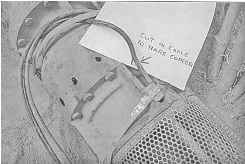
FIGURE 5 A submersible pump bowl perforated in several locations as a result of stray current emanating from a damaged power cable
