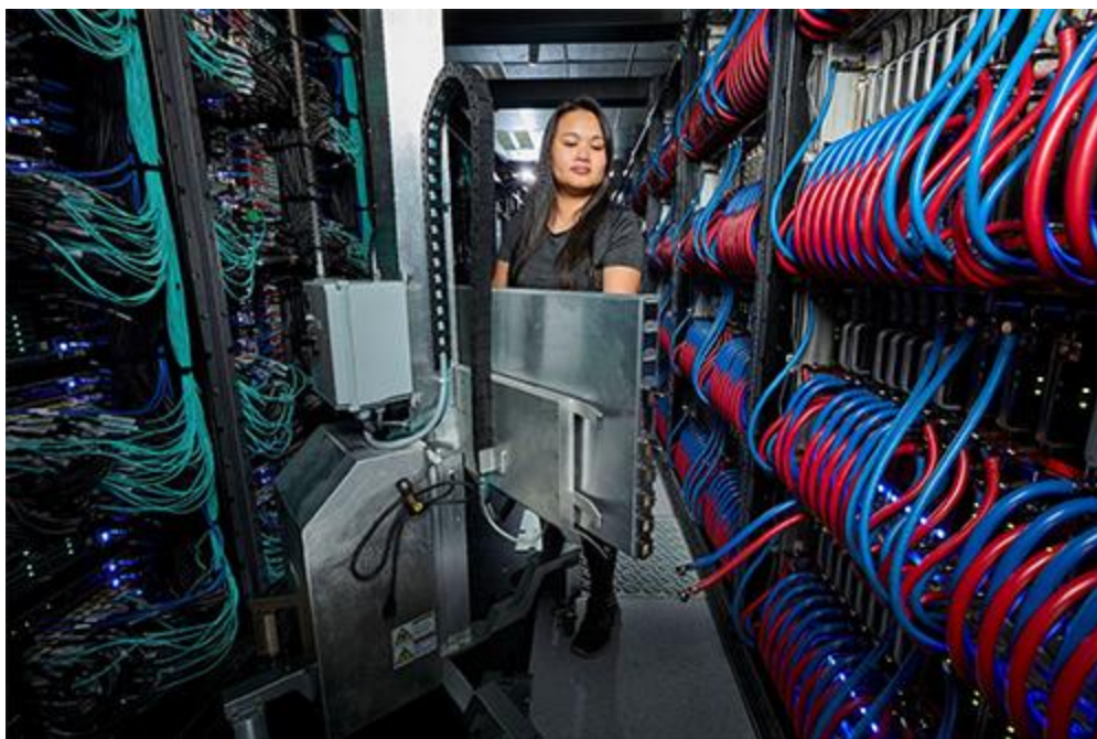
Lawrence Livermore National Laboratory technician Ty Nguyen works on installation and maintenance of El Capitan’s compute blades.
