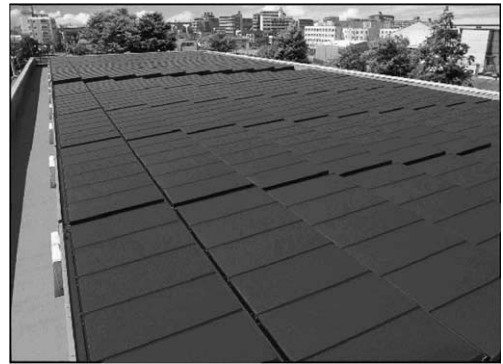
Fig. 20. KW system at the top of the building Osaka (HYBRID modules). Note that modules are installed at low angle (5 degree off from horizontal).
