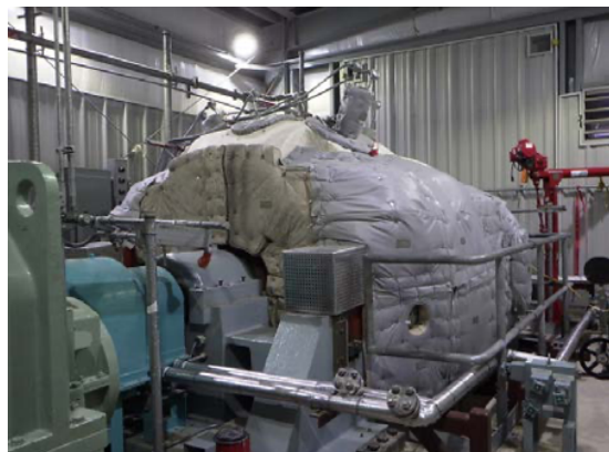
Figure 2: Installed Turbine at demonstration Plant
