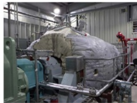
Figure 2: Installed Turbine at demonstration Plant
