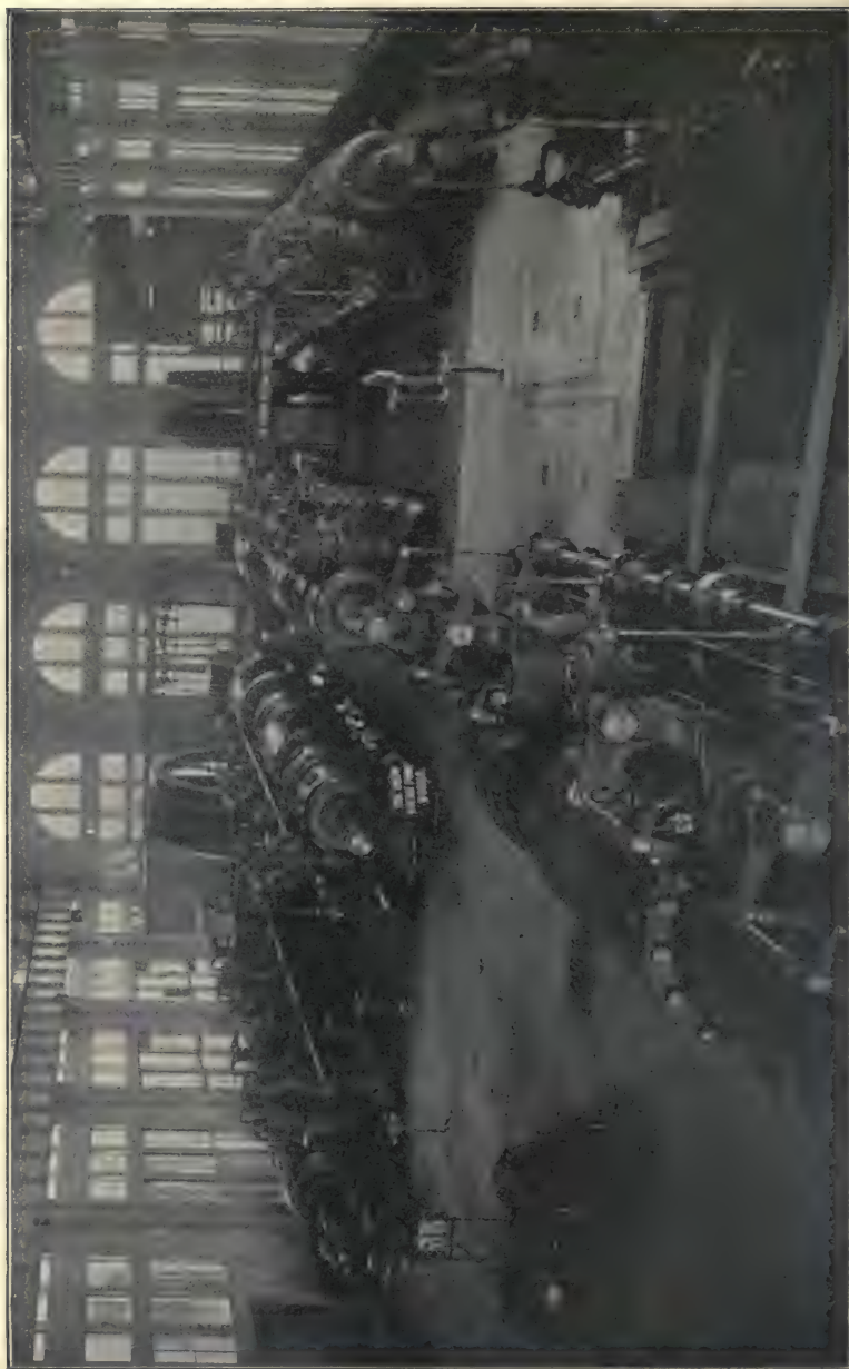
Fig. 12 74. — Snow Type A Engines, Martin Station, San Mateo Power Co., Cal.
