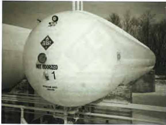
EXHIBIT 5.18 ASME Containers Marked NOT ODORIZED.
