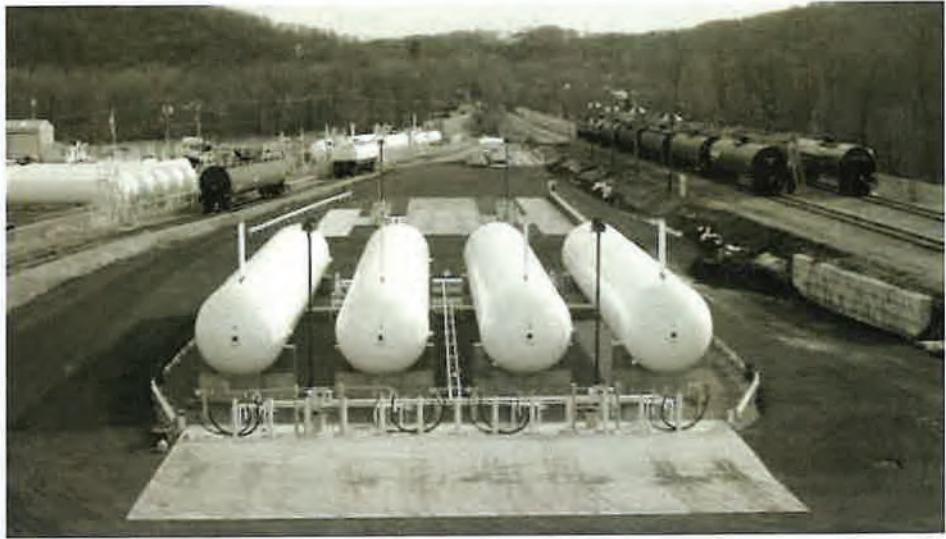
EXHIBIT 3.3 Large Bulk Plant. (Courtesy of Eastern Propane Corp.)
